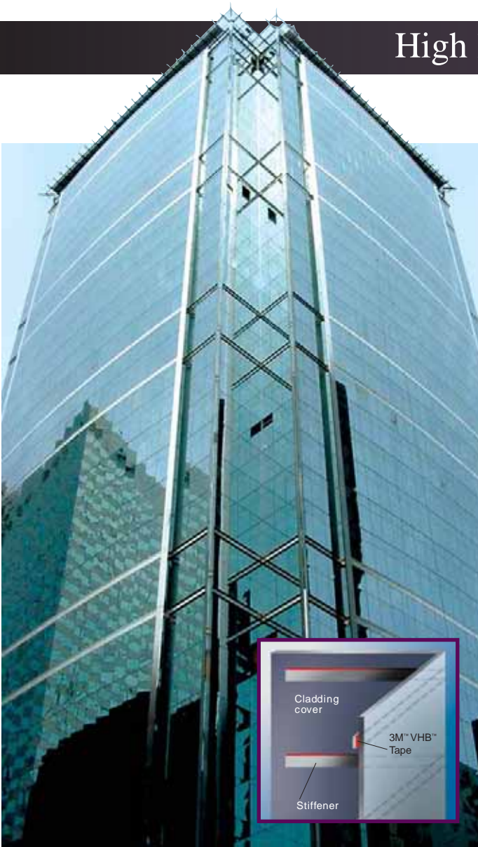
Dearborn Center, Chicago, IL, USA Fabricator: Copper Sales Una-Clad, 2003 Stiffeners bonded to exterior metal trim cladding.
